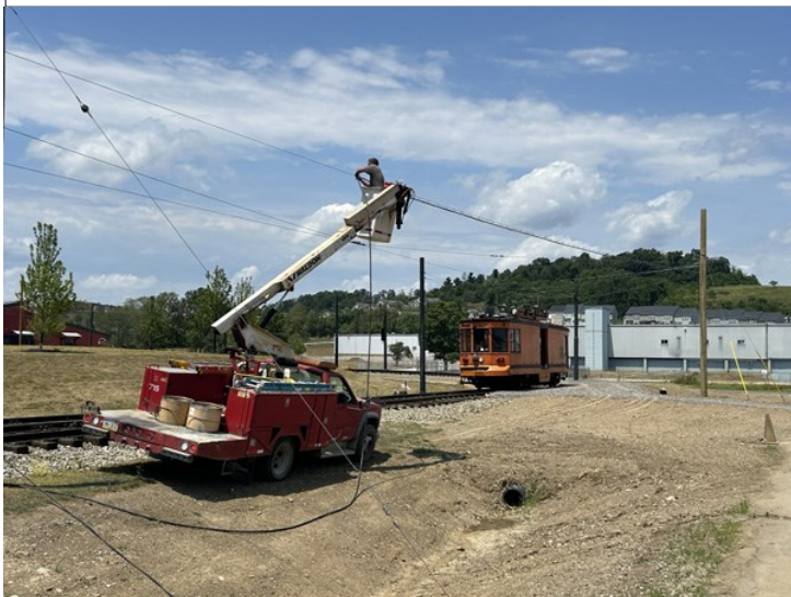
Kevin and volunteers install wire for lights at Ellis Stop 7-15-24. Scott Becker photo
