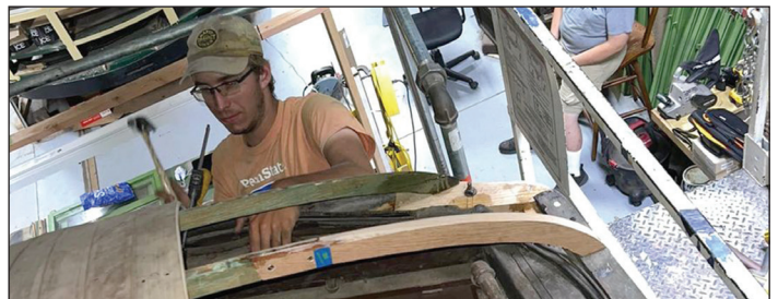
Michael Buchta spearheaded roof bonnet repair on Red Arrow car 73 with help from many of our other younger volunteers including CJ Bick during work on both ends of car 73. Laura Wells photo
