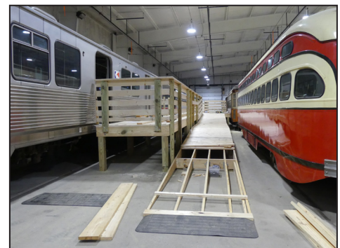
In March the crew from the Washington County Correctional facility started construction on the high platform at the Display Building. Bruce Wells photo
