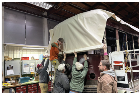
Canvas initial roll out onto the roof of PST 73. Scott Becker photo
