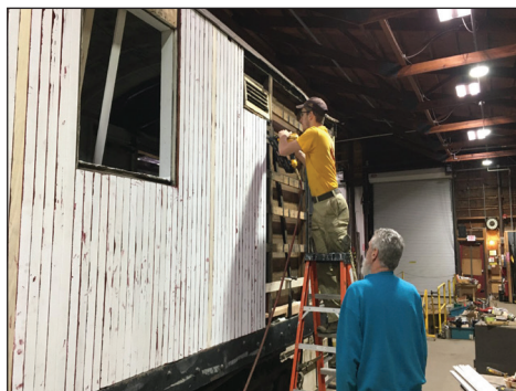
Buck and Michael installing new wood siding on P&WCTCo O7 in preparation for it's display on the right of the platform shown here. Scott Becker photo
