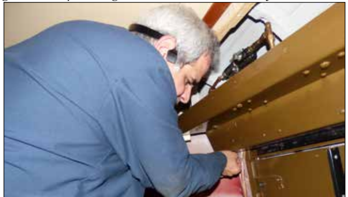
Art Rizzino finishes up the piping for the door engines with protective sleeves to guard against wear to the pipes in 832.
