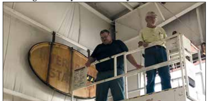
Jeff King and Scott Davis work from the scissors lift at the TDB to install the Washington Interurban Station sign.
