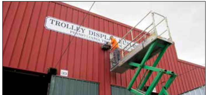
Rich Kliza of R.K.E.S. LLC removing old lighting fixture at Trolley Display Building Photo by Scott Becker
