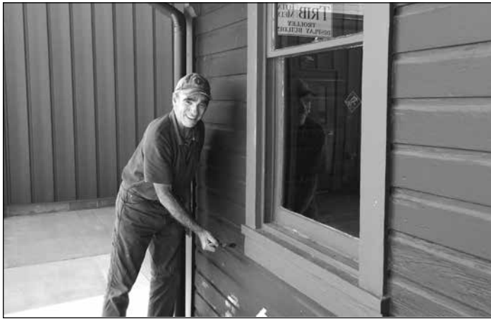
Larry Lovejoy puts finishing touches on the Wexford Station Photo by Bruce Wells
