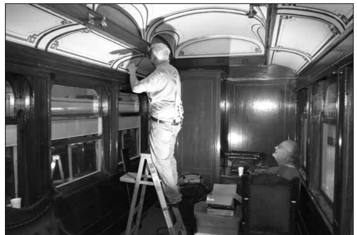
Bill Fronczek and Fred Cooley working on the wiring inside the private car Toledo. Photo by Bruce Wells
